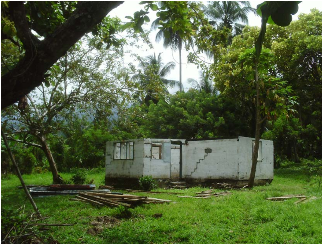
Figure v. Old techers house built in 1962, beyond repair
